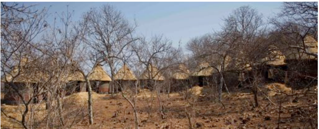
Rondavels under construction for the childrens’s bush camp to host 4 day conservation camps
